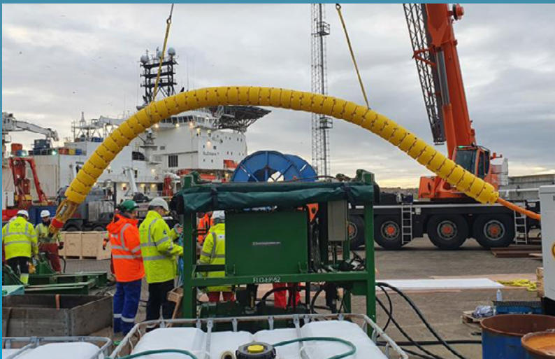
Installation of Subsea Energy Solutions' Sub-VBRTM vertebrae system onto a cable at quayside.
