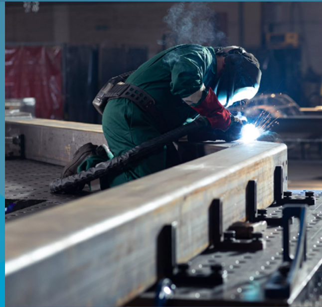
Box section steel welding Image courtesy of Hutchinson Engineering. All rights reserved.
