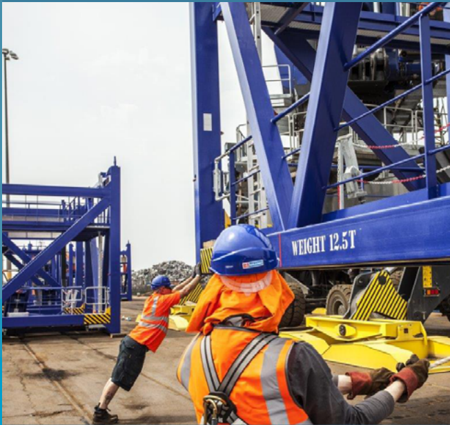
Internal platform module being lifted. Image courtesy of Hutchinson Engineering. All rights reserved.
