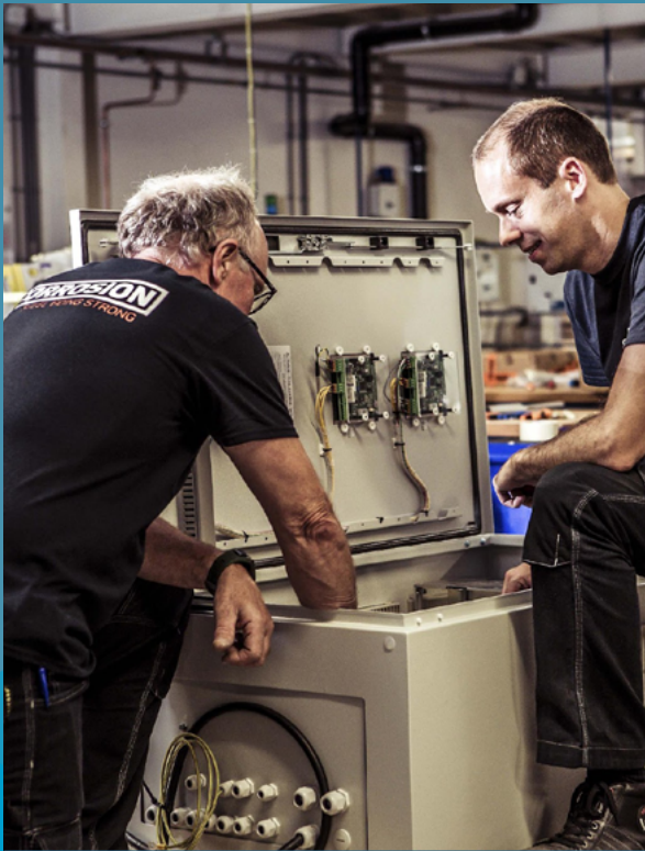
Assembly of a power cabinet. Image courtesy of CORROSION. All rights reserved.
